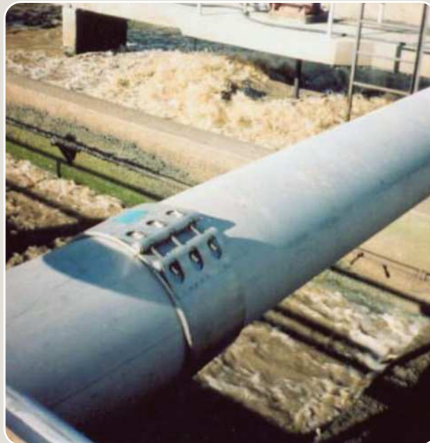
▲ Spain: water purification facilities
