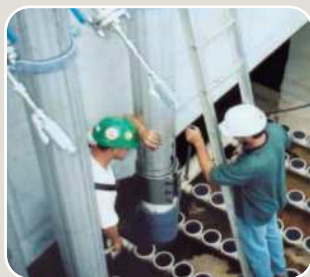
▲ Canada: water purification facility
